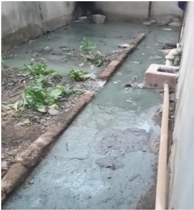
Figure 1. Sewage spills at one house in Chegutu town
